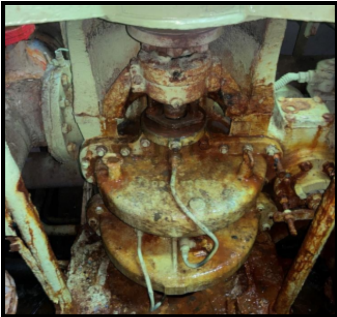
Corrosion and leakage of main fire pump
