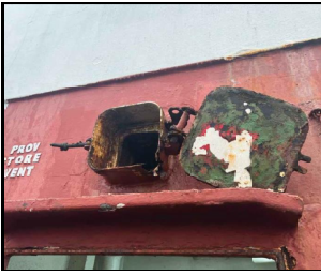
Corrosion of natural ventilator
