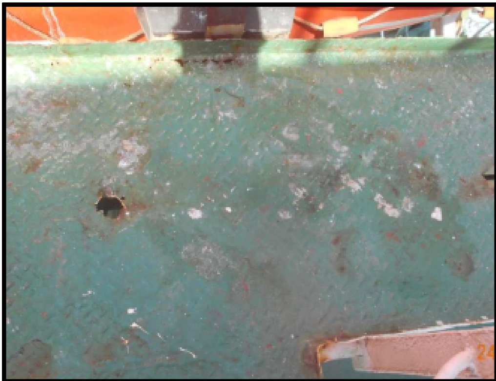
Holes on lifeboat embarkation station platform
