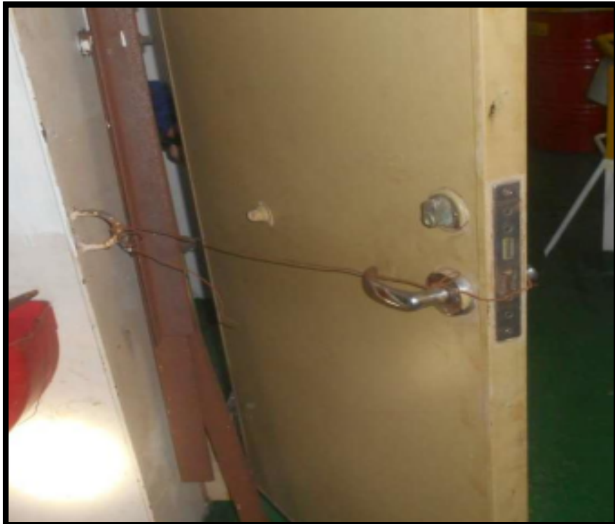
Hold-back wire attached to fire door
