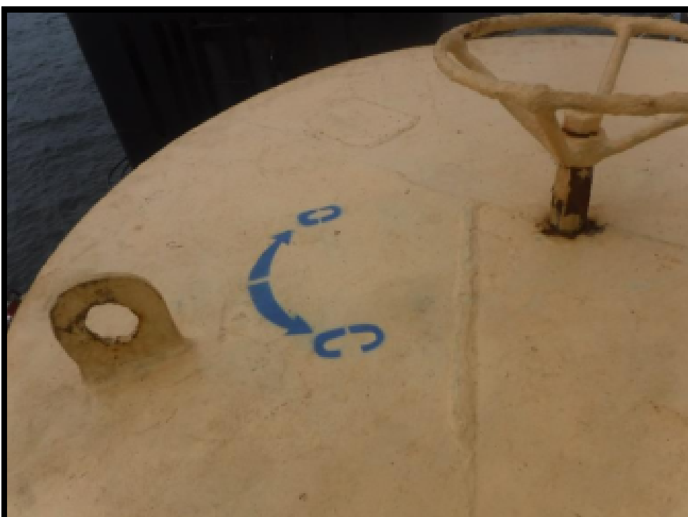
Incorrect marking of ventilation open/close direction
