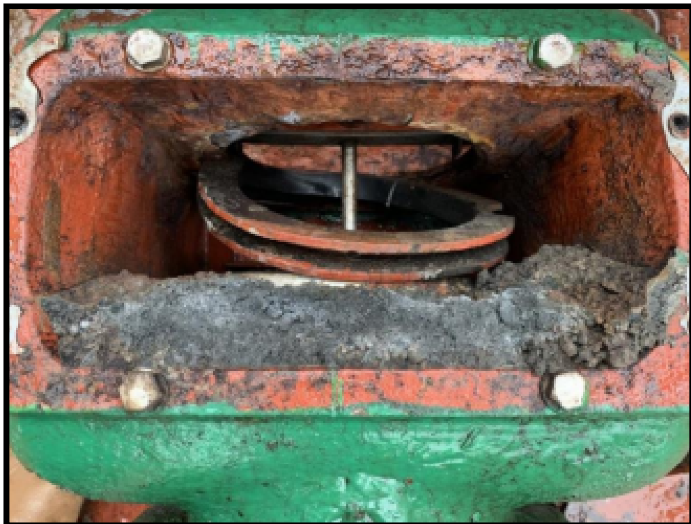
Defective air pipe head fittings
