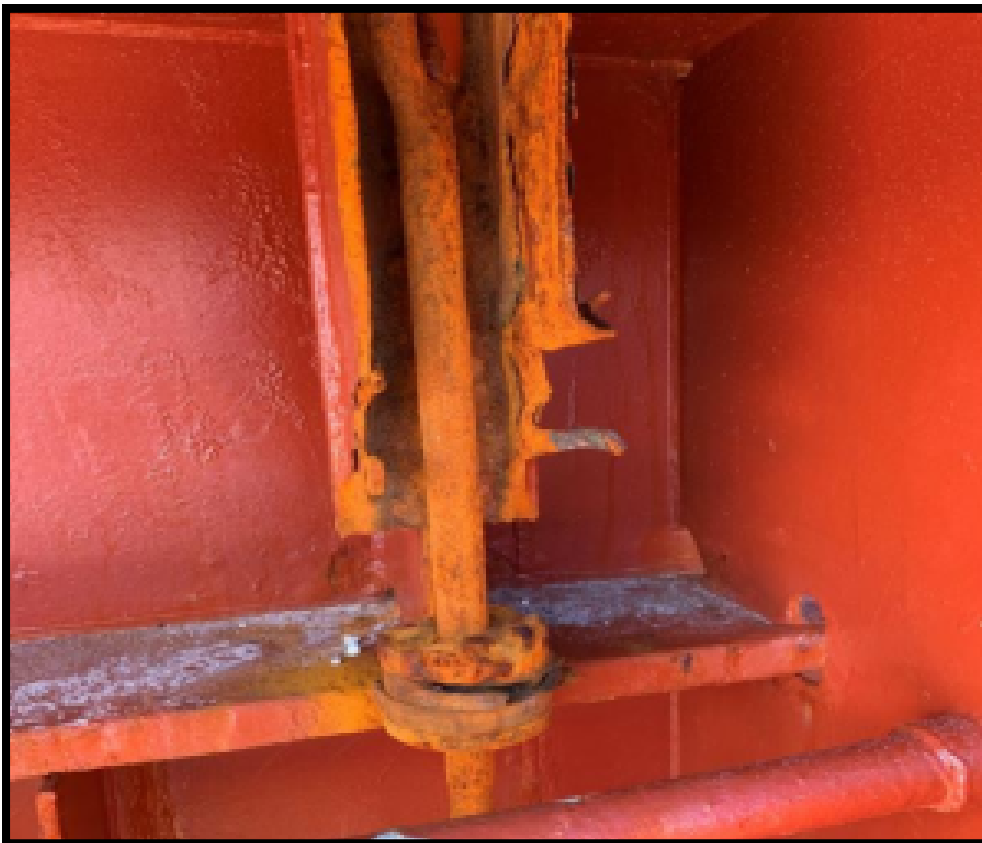
Corrosion of hatch cover cleat
