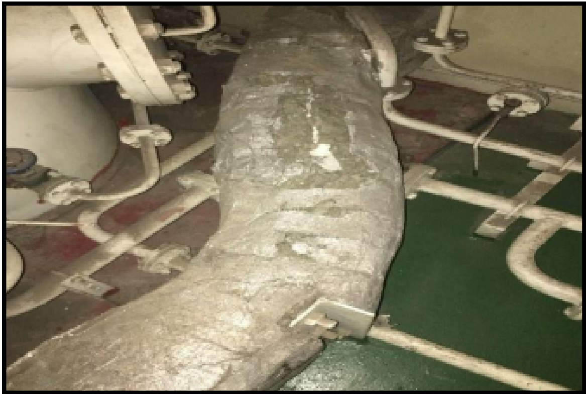
Damage to insulation material for fire line suction pipe (passing through engine room)
