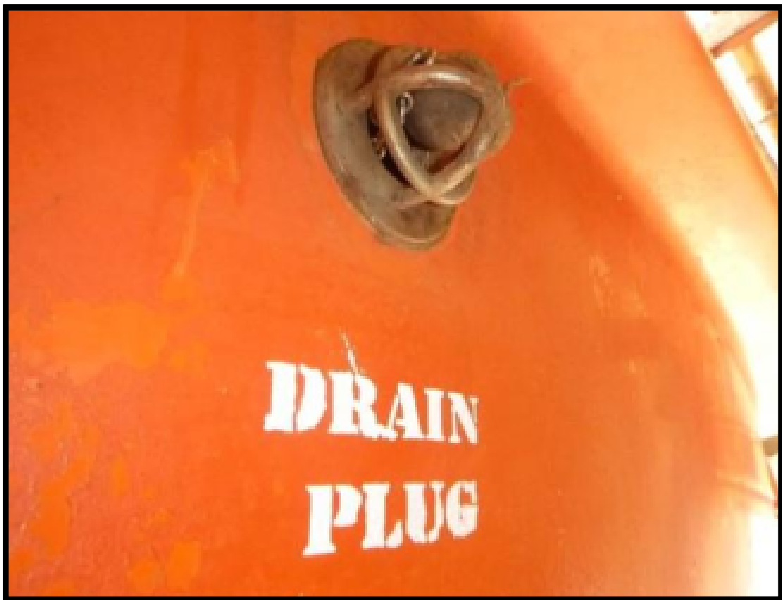
Deterioration of lifeboat drain plug (rubber ball)
