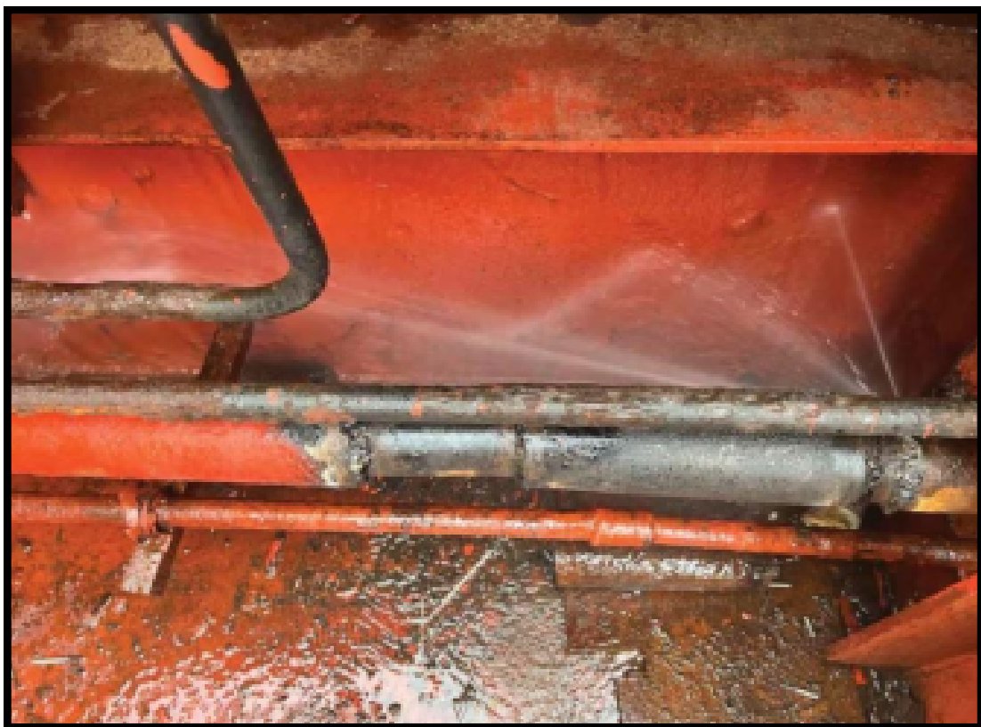
Leakage of fire line
