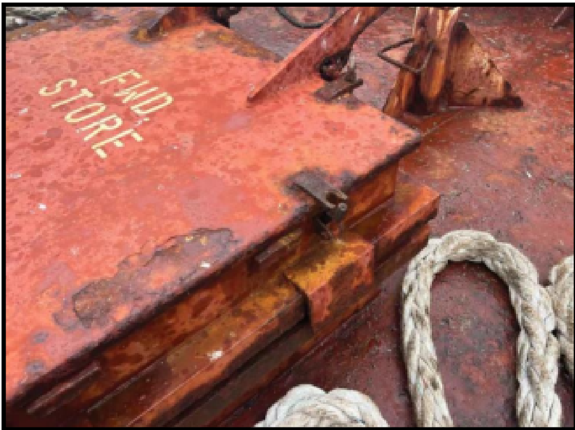
Access hatch closing bolt partly missing
