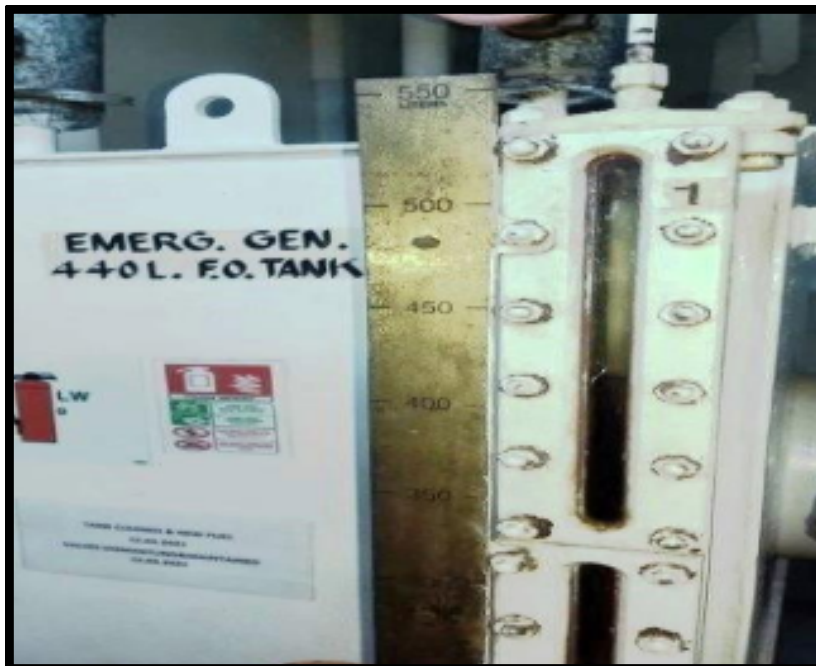
Insufficient diesel for emergency generator
