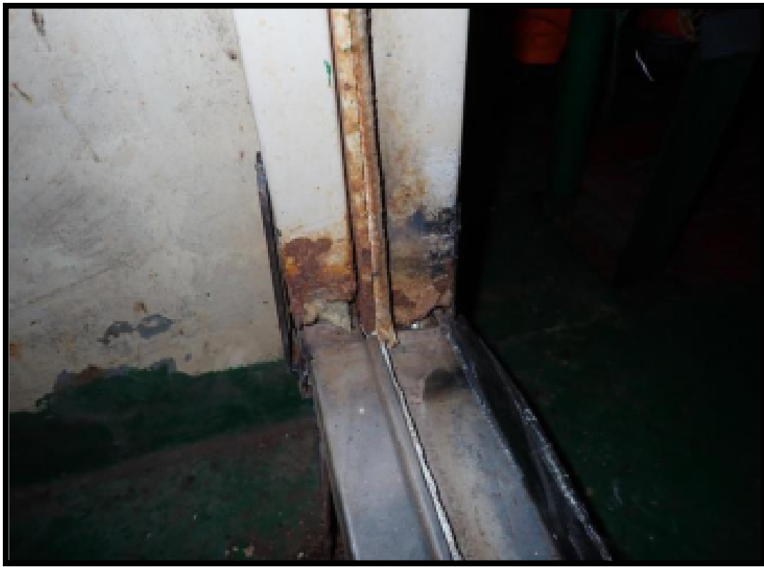
Corrosion of fire door and door frame
