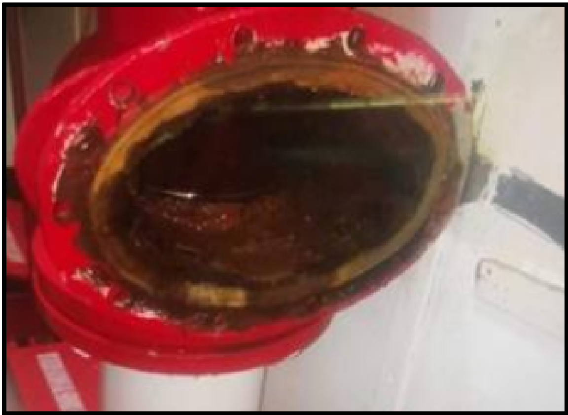
Malfunction of fire line isolation valve due to mud
