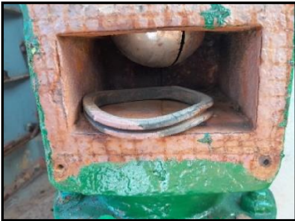
Broken float/worn out rubber packing of the air pipe head
