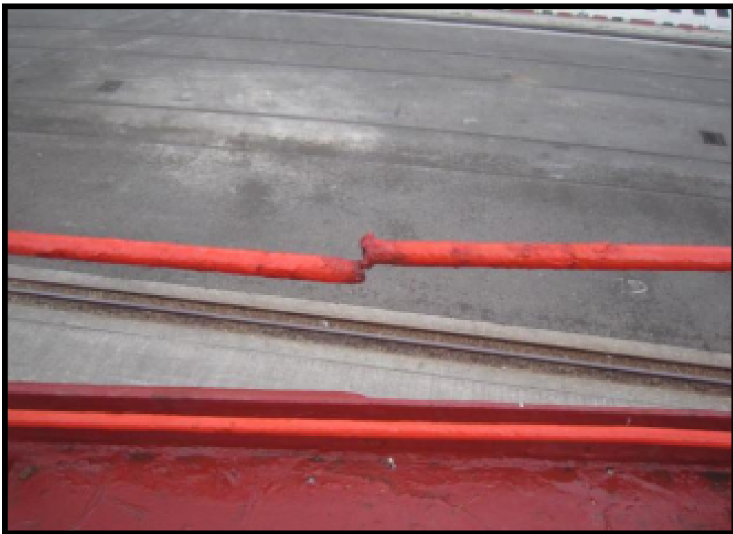
Damaged guard rail
