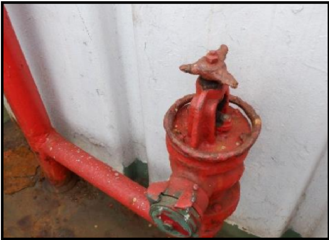
Broken hydrant handle
