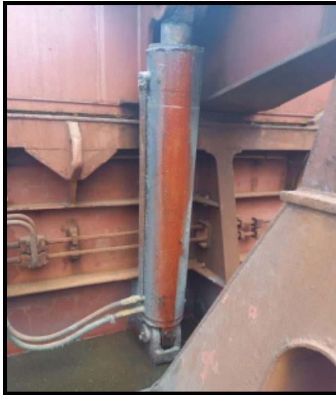
Oil leakage from hydraulic piston for hatch cover
