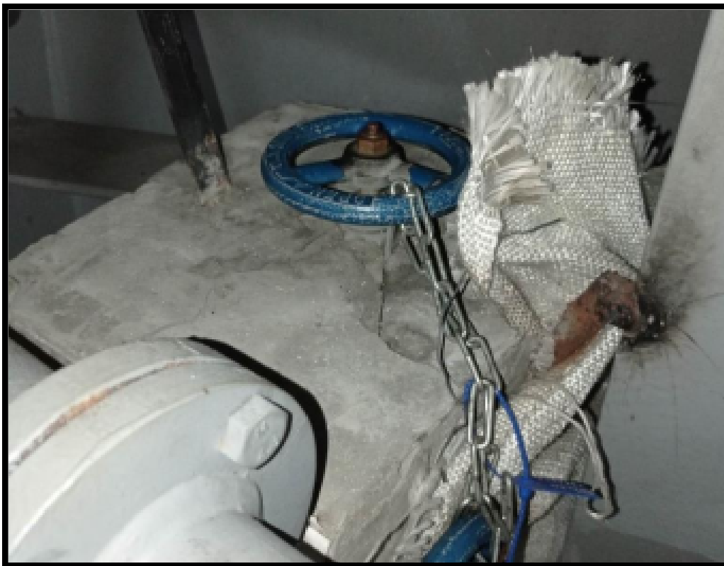
Unreported temporary repair with cement box to RO
