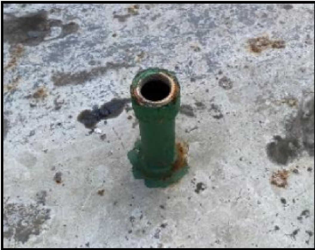
Missing sounding cap
