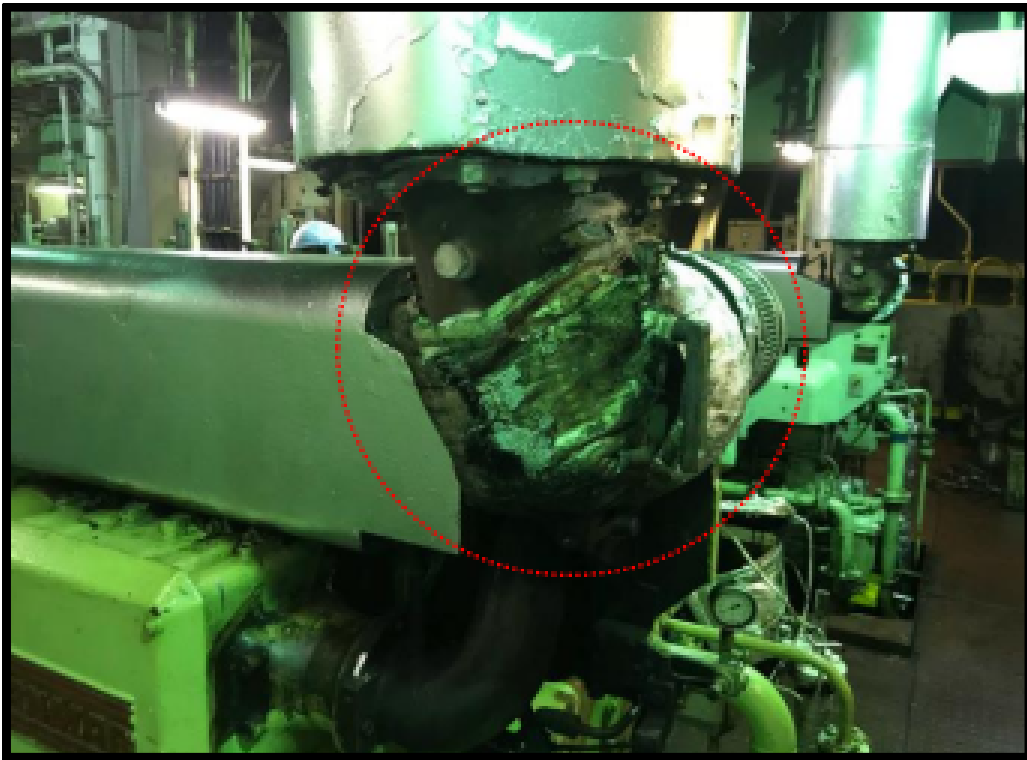
Deterioration/peeling of insulation on exhaust pipe of M/E
