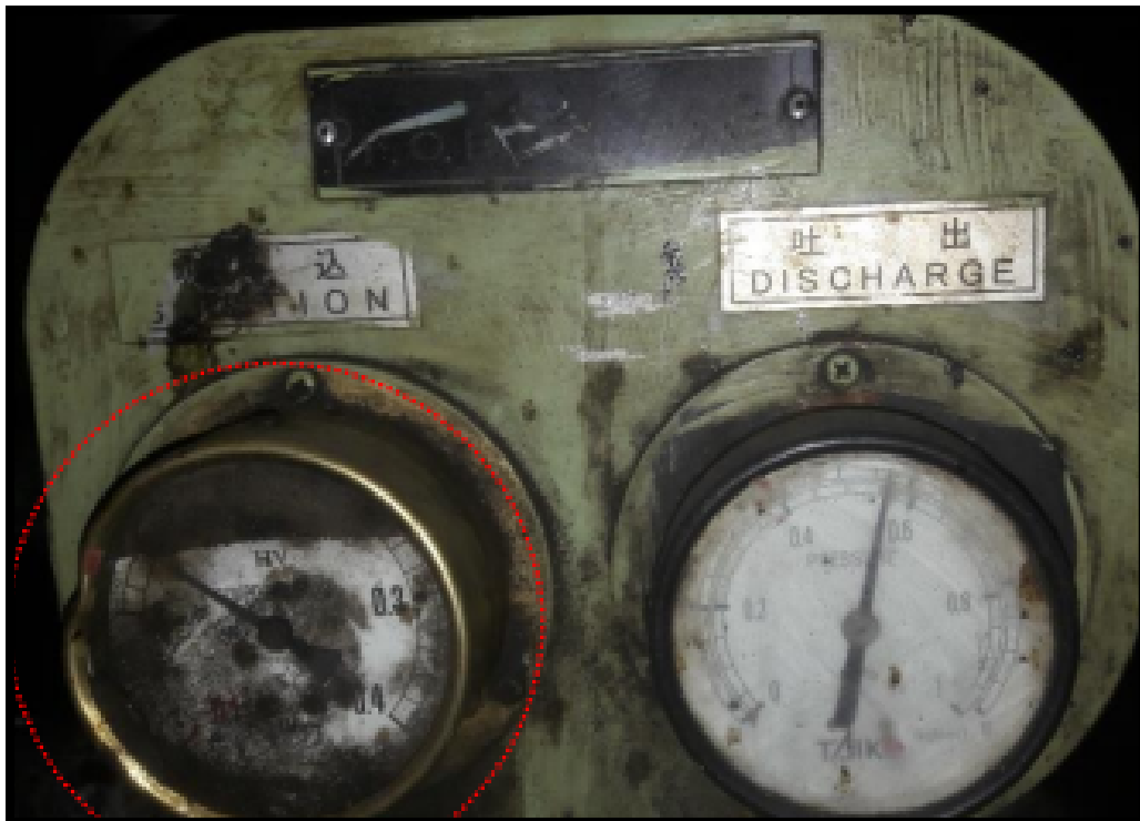
Defective pressure gauge of FO pump
