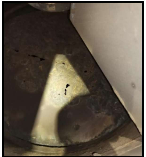
Corroded/holed fire damper for E/R
