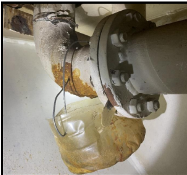
Leakage from pipeline
