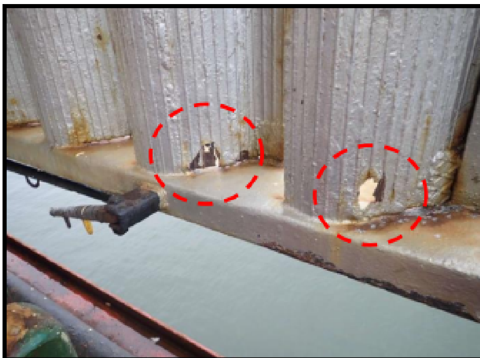
Damaged life buoy
