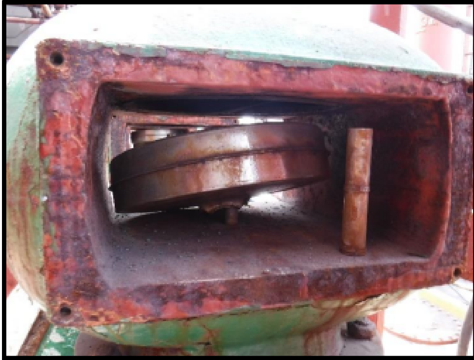
Broken float disc of the air pipe head
