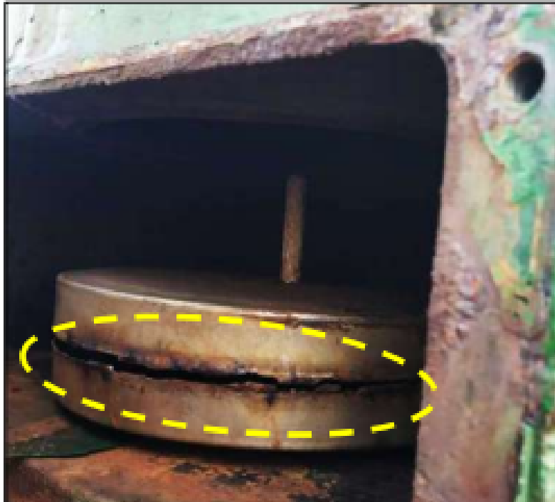
Broken float disc of air pipe head
