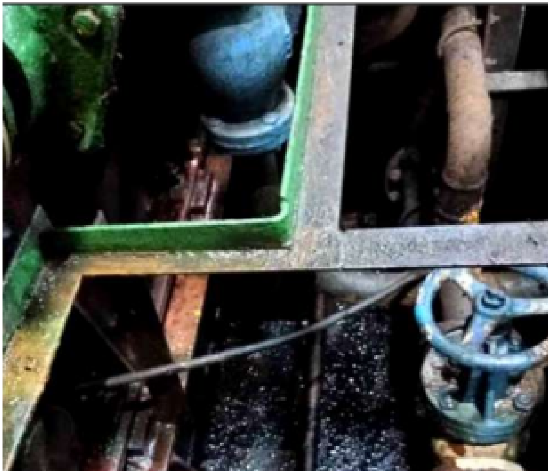
Dirty condition in engine room
