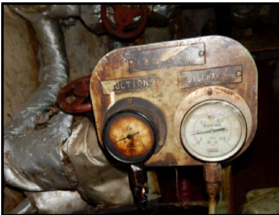
Dirty pressure gauge
