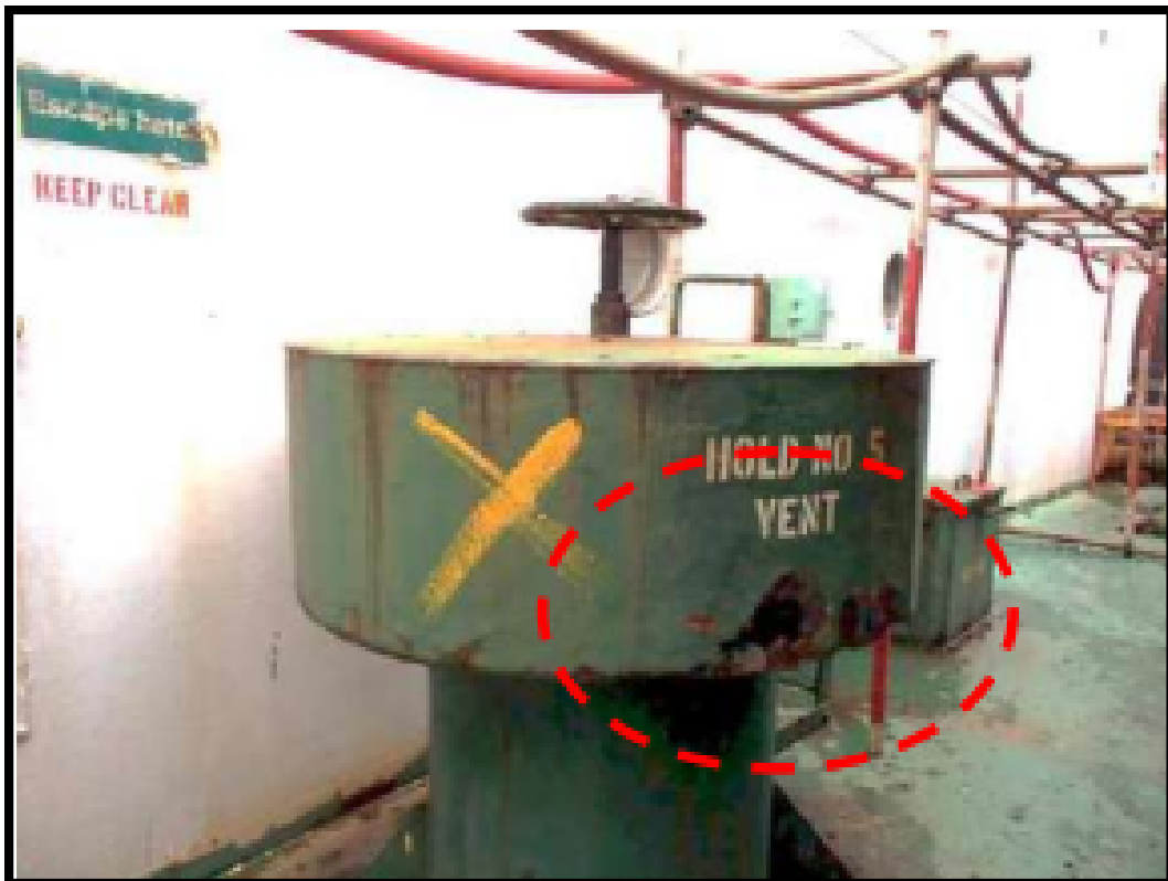
Holed mushroom ventilator
