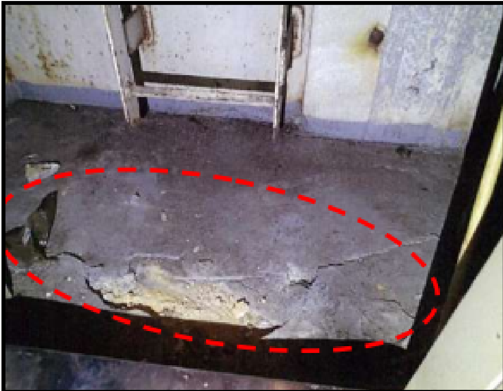
Fractured escape trunk bottom
