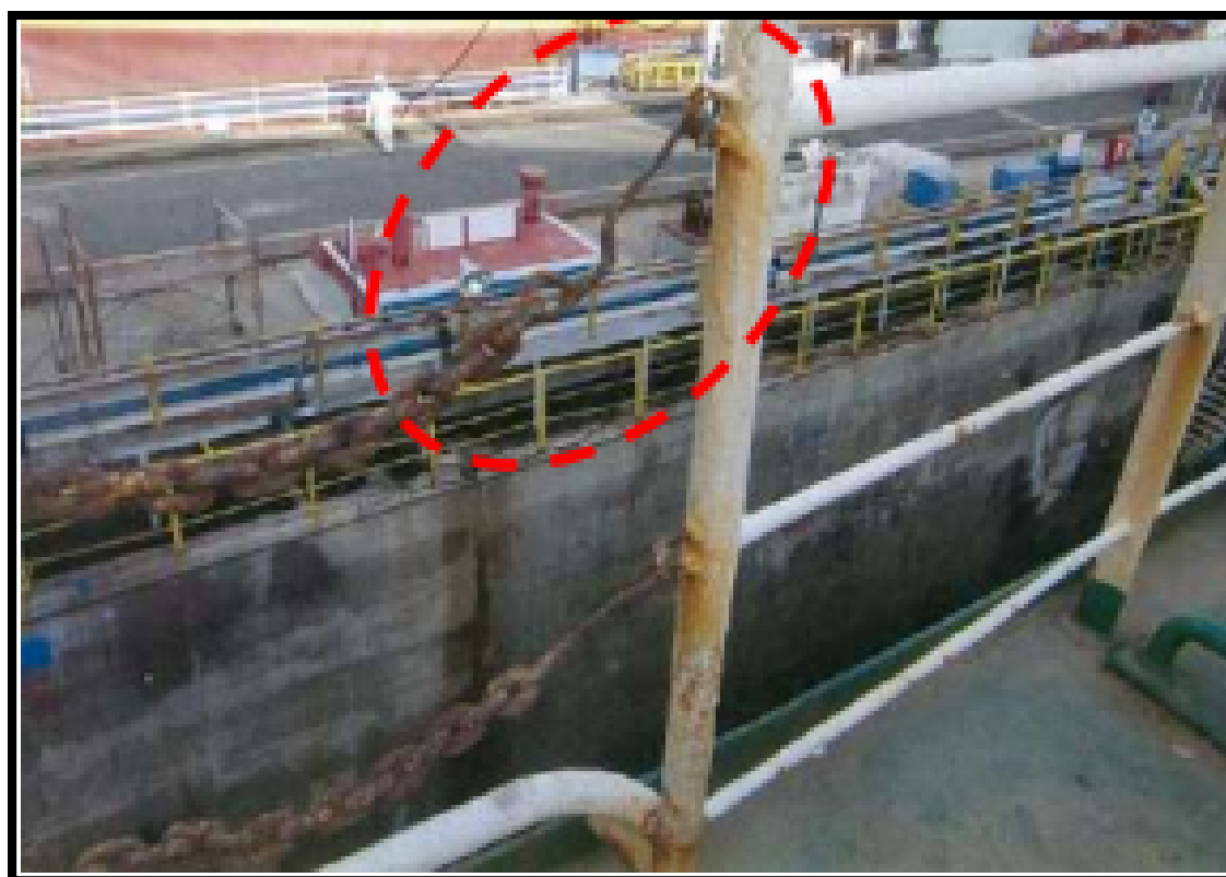
Improper chain hook
