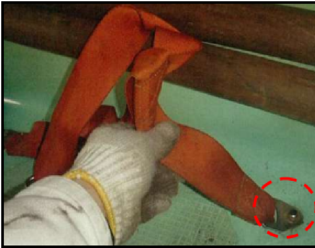
Loose foundation bolts for seat belts
