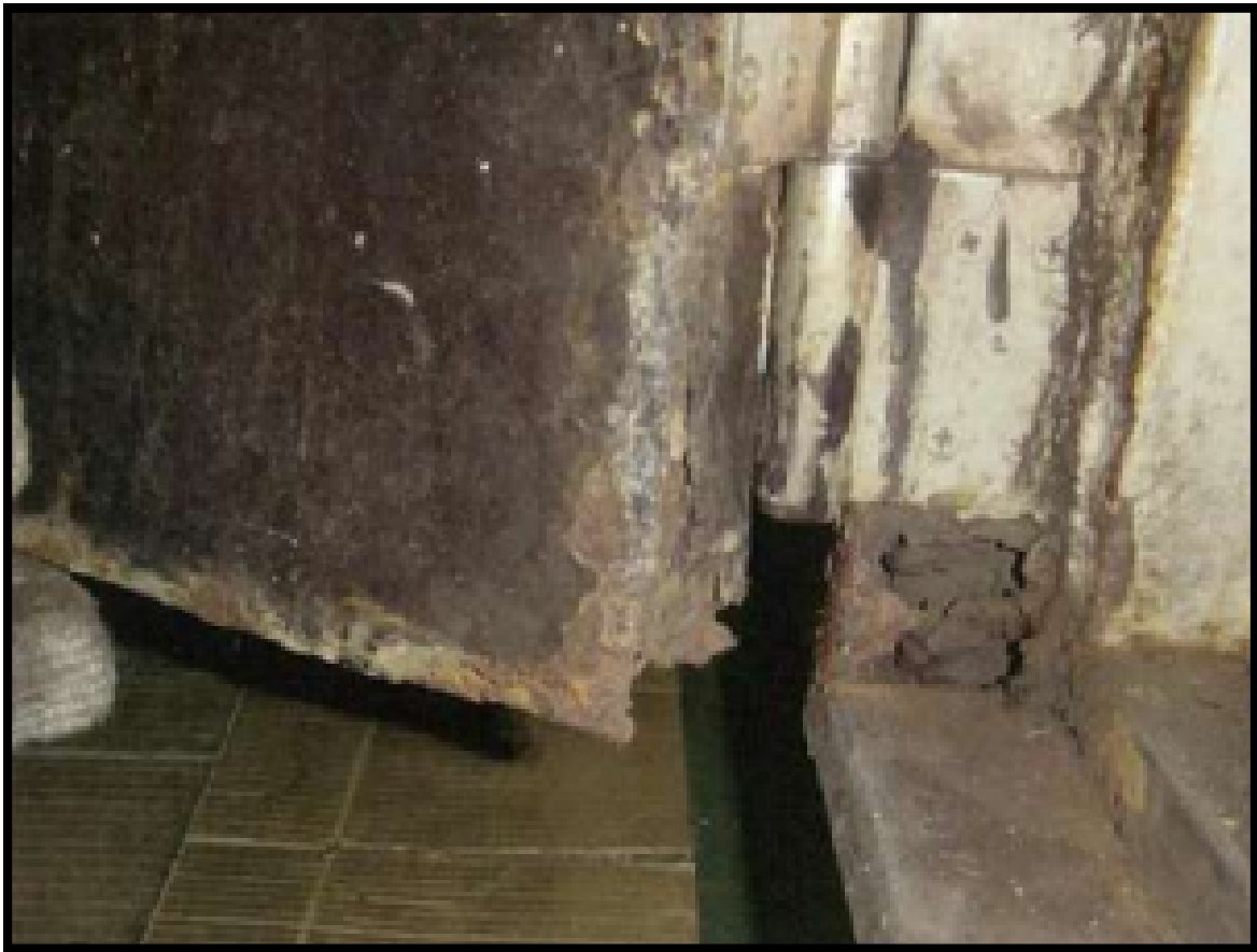
Wasted fire door and its frame
