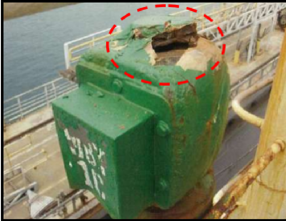
Holed air pipe head
