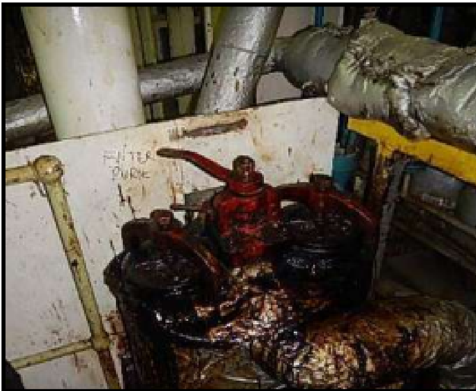
Oily and dirty engine room
