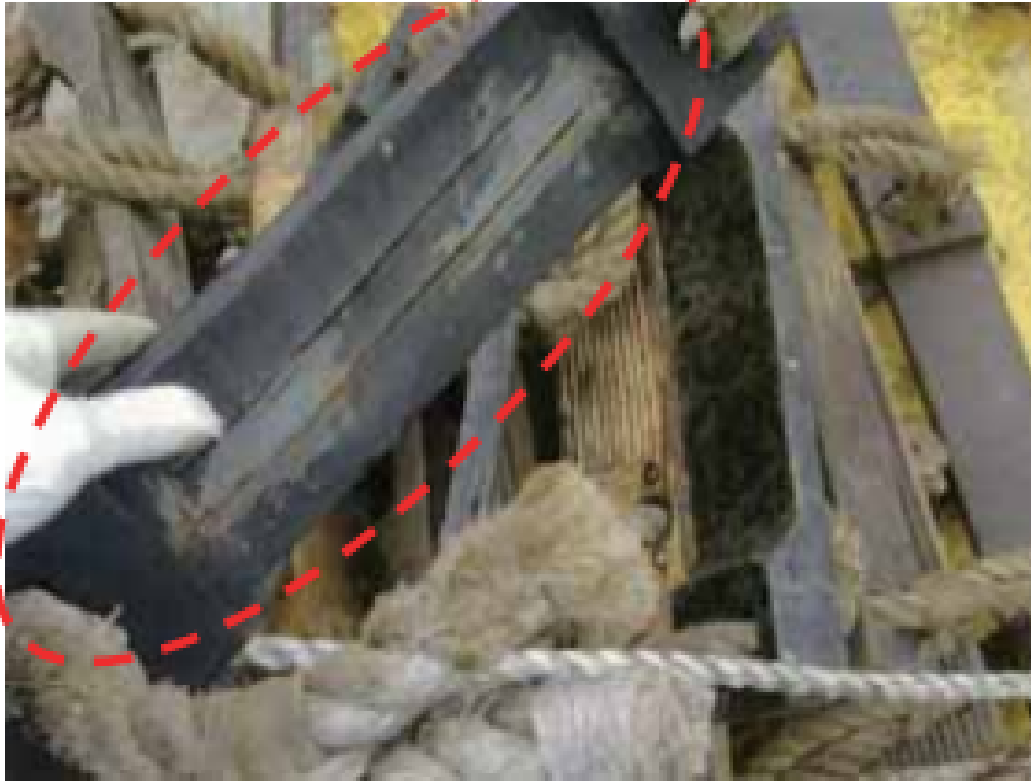
Poor condition of embarkation ladder
