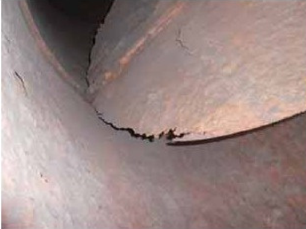
Wasted fire damper flap
