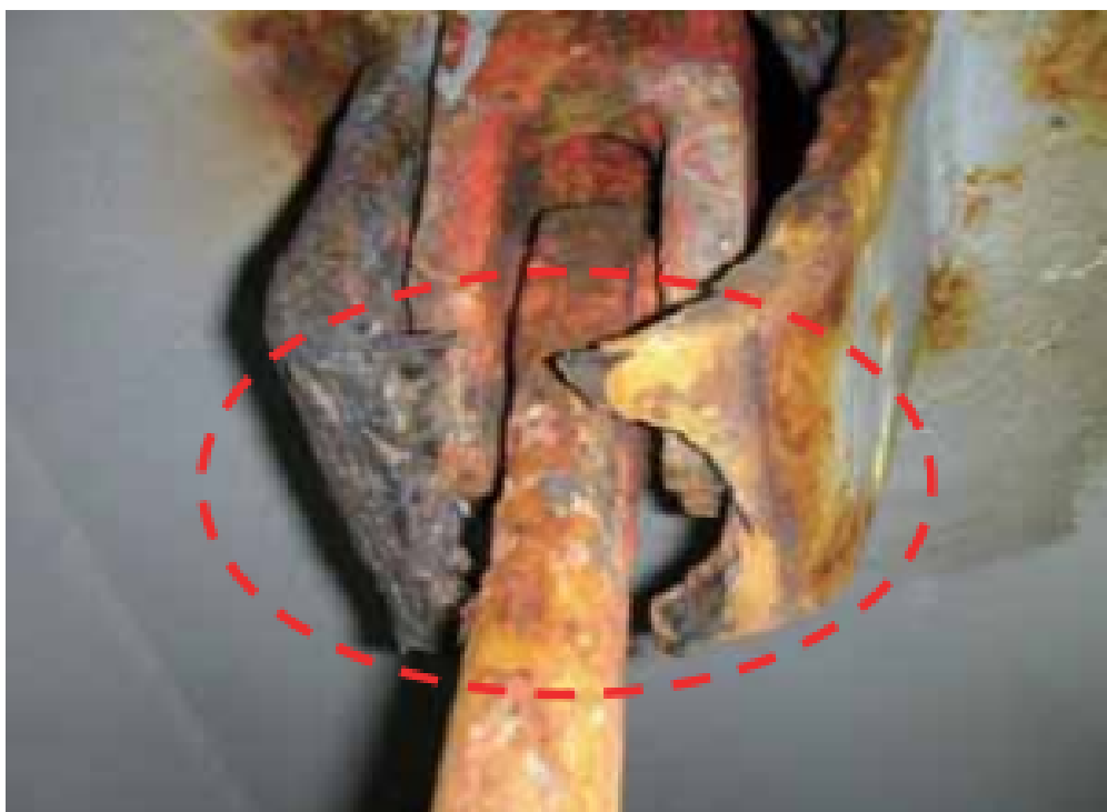
Wasted and corroded hatch cover securing device
