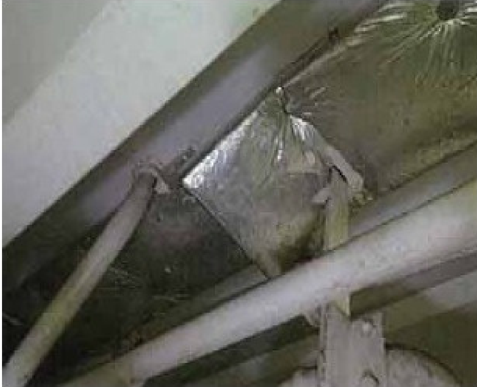
Detached insulation on underside of deck
