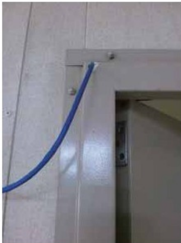
Improper cable penetration (through fire door frame)
