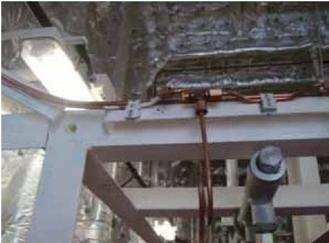
Disconnected pilot line for fixed CO2 fire extinguishing system
