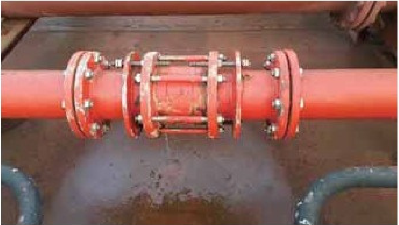
Leakage from fire line
