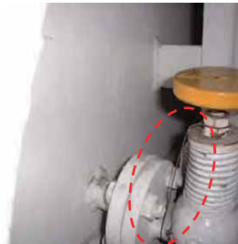
Emergency shut-off valve not ready for use (secured by wire)
