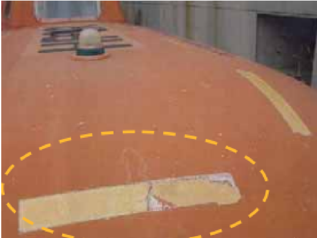
Deteriorated reflective tape
