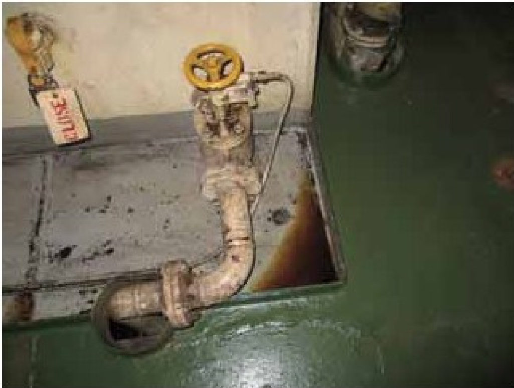
Oil leakage and accumulation
