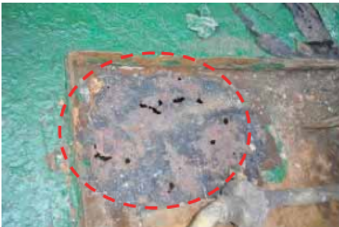
Corrosion holes on strength deck
