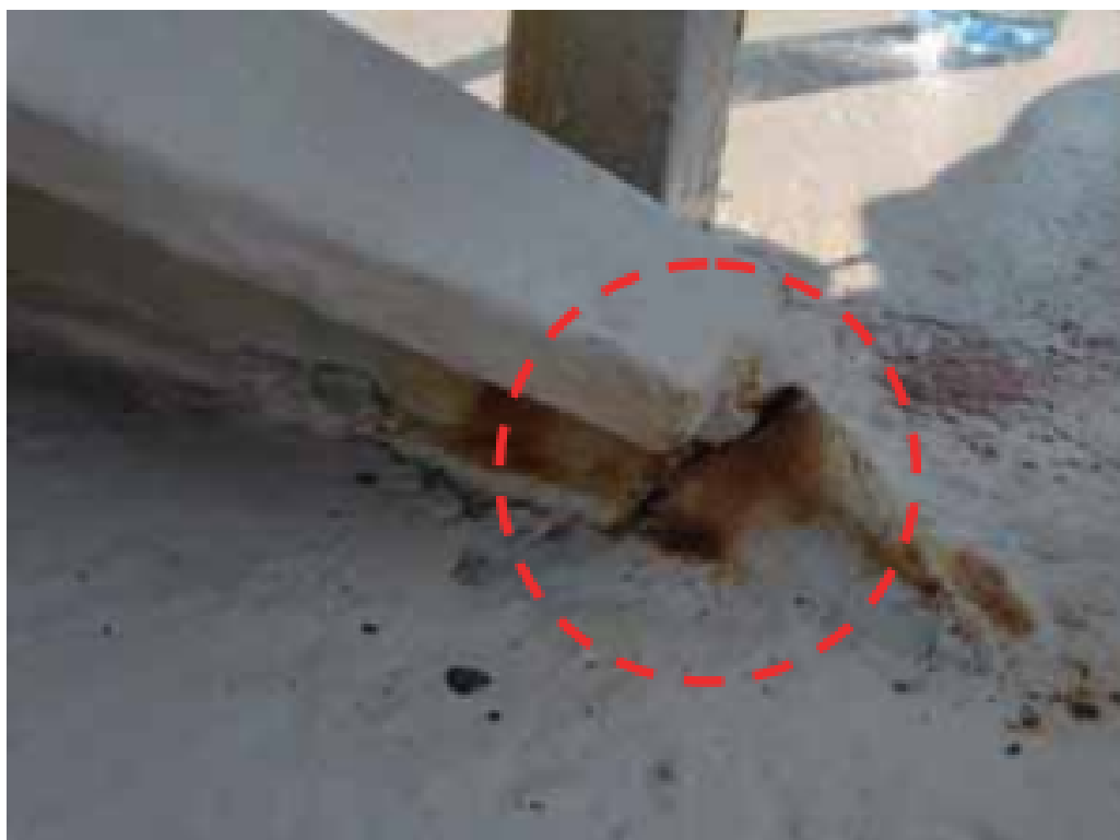
Crack at toe of hatch side coaming end bracket
