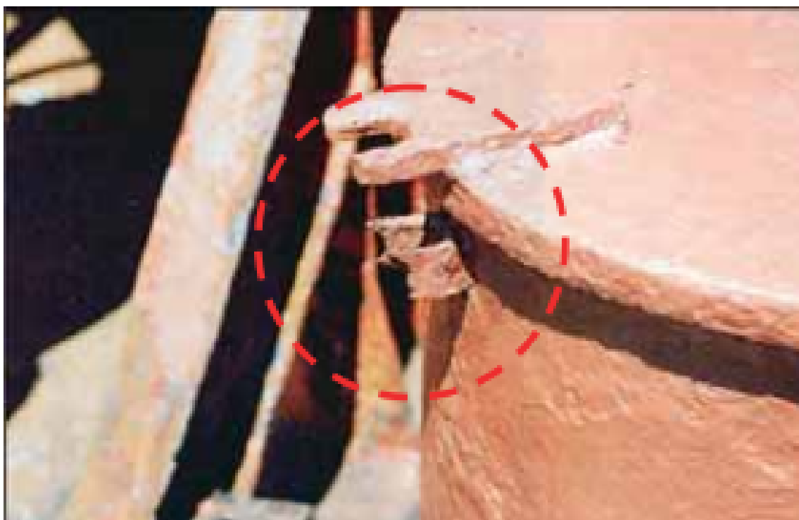
Missing of hatchway securing device
