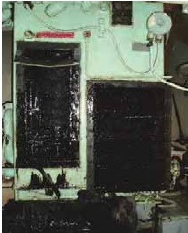
Clogged oil water separator
