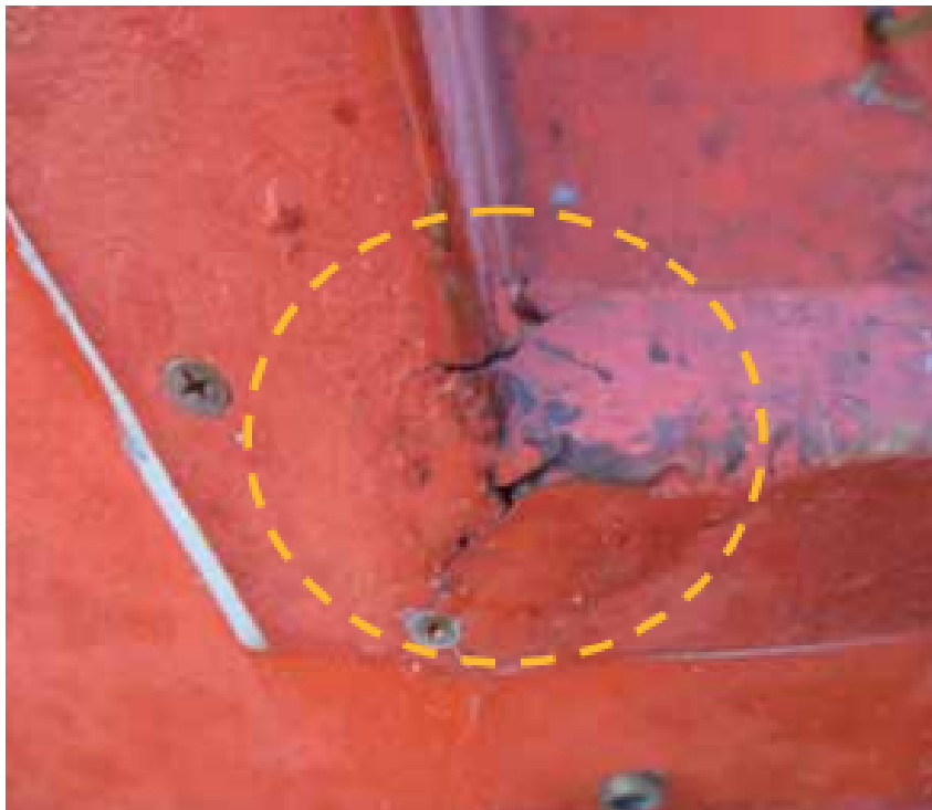
Fractures on lifeboat hull
