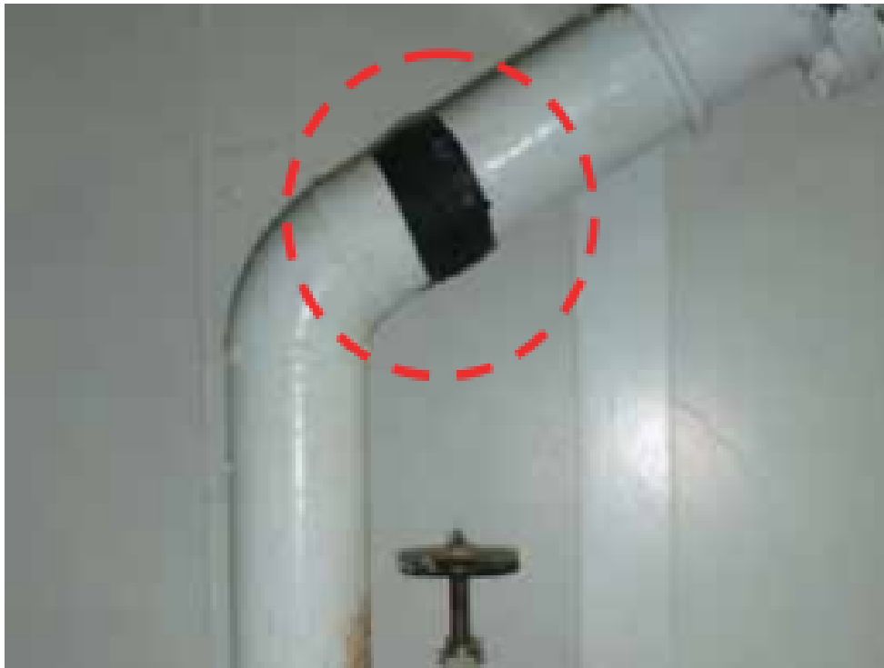
Pipe temporarily repaired with rubber patch
