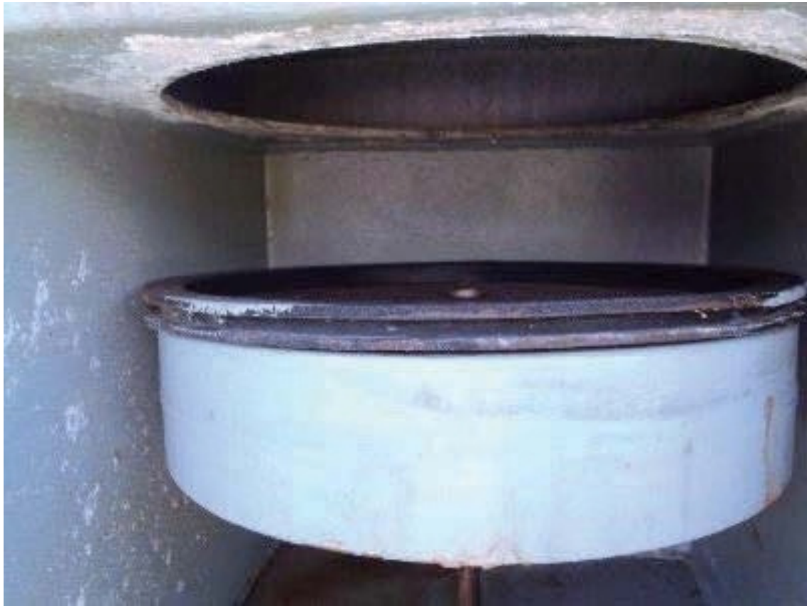
Detached gasket of cargo hold air vent
