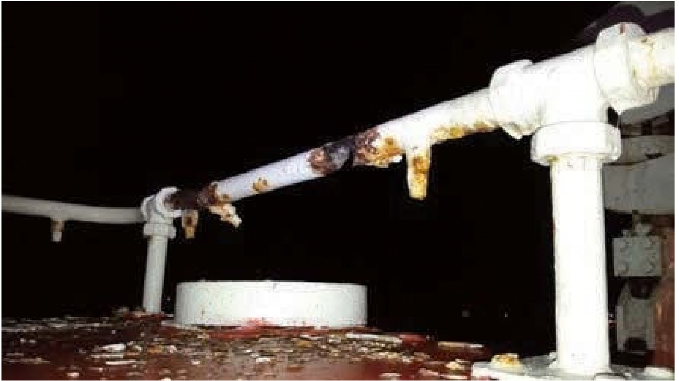
Corrosion and Hole of water spray
