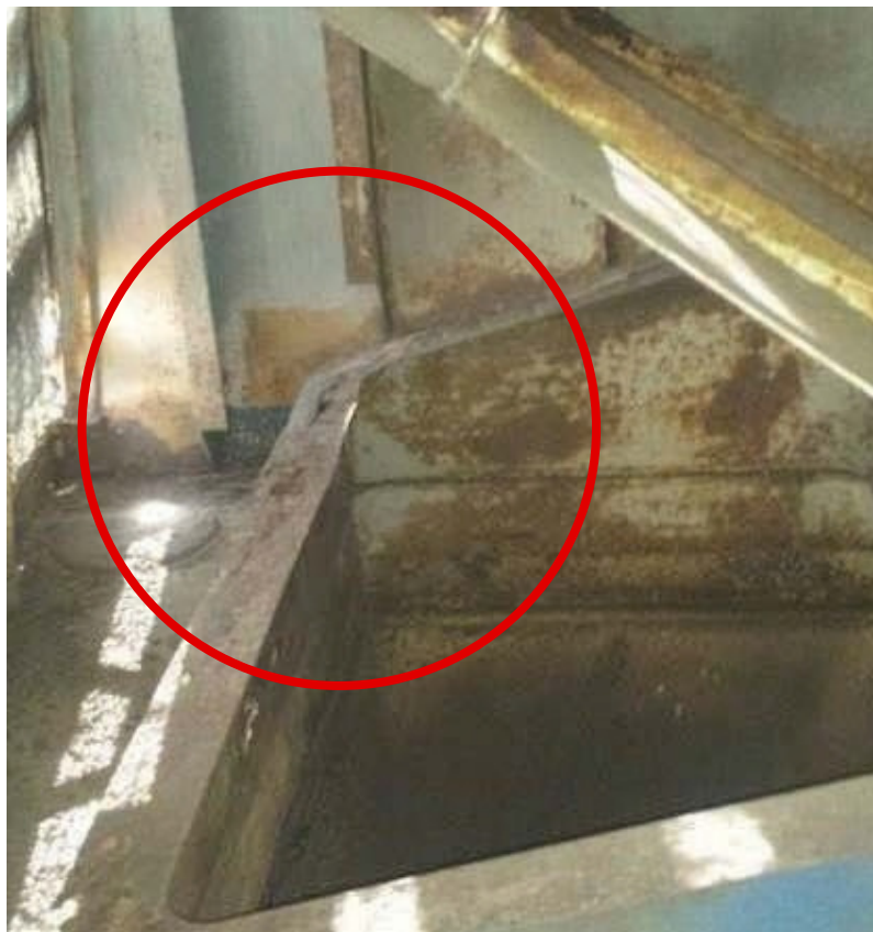
Holed funnel ventilation
