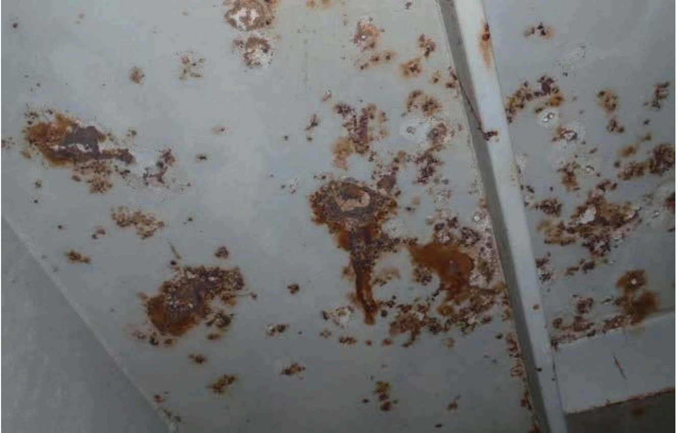
Corrosion holes of strength deck
