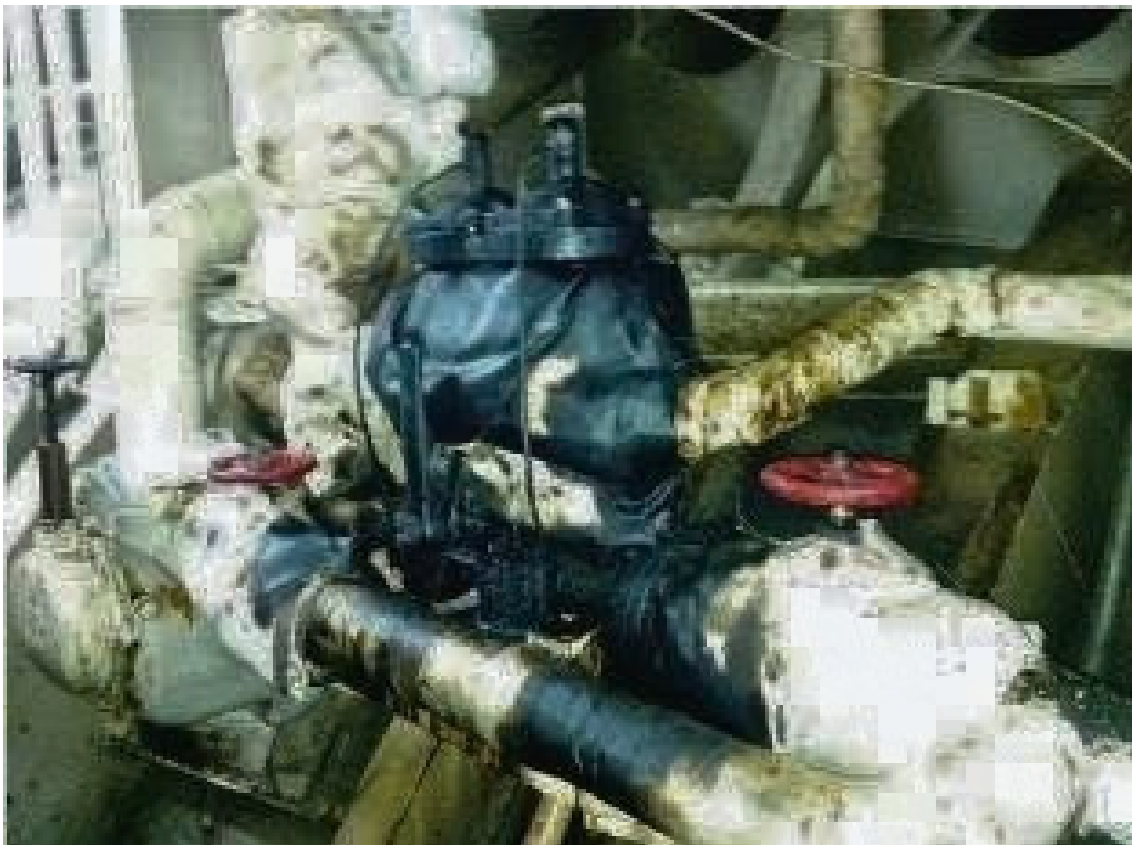
Oily lagging of F.O. piping
