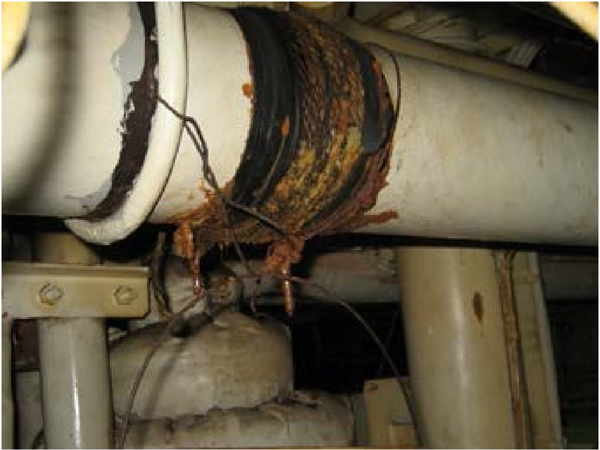
Patched sea water pipe
