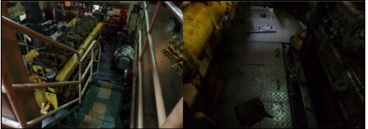
Oily, unnecessary items scattered engine room
