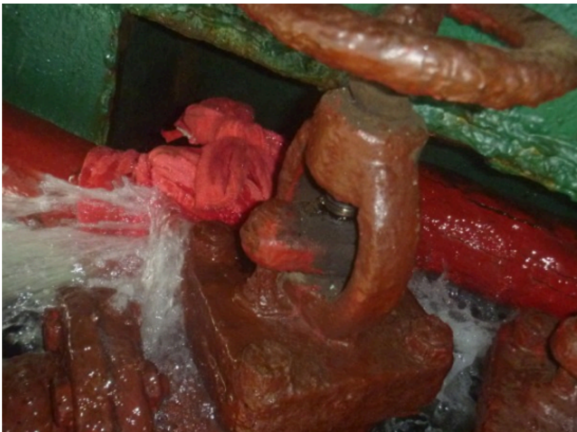
Fire main pipe leaking during testing
