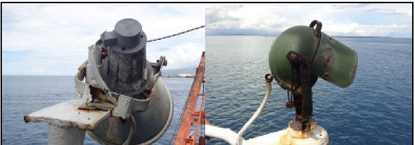
Open / Not secured electrical wires hazard
