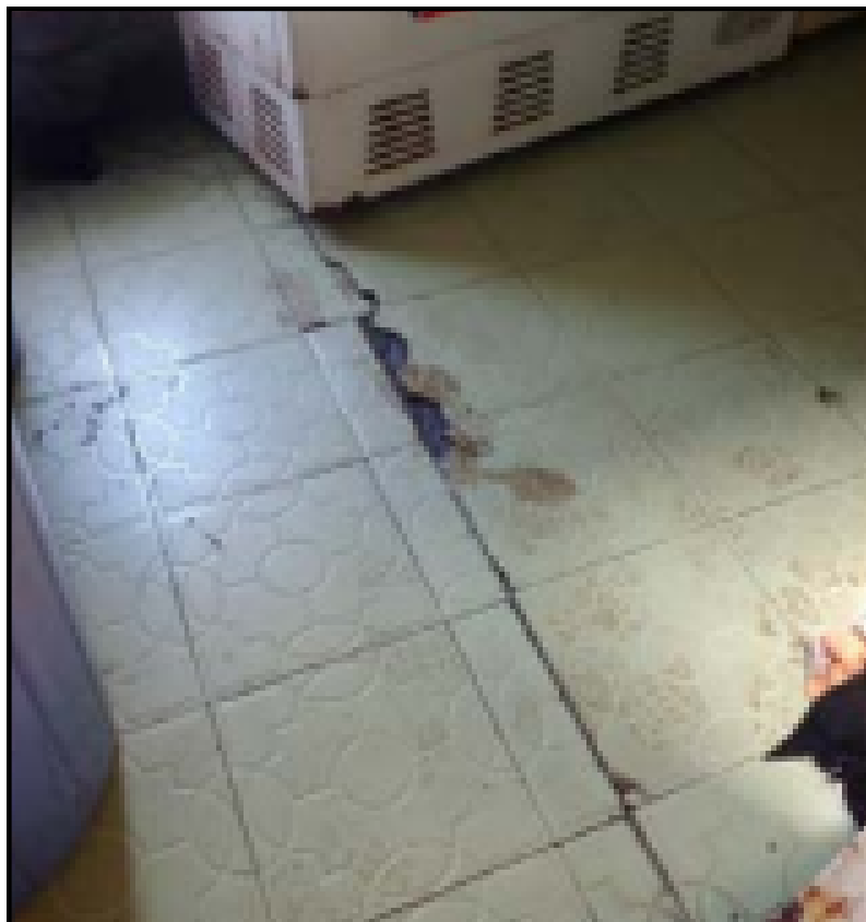
Deteriorated vinyl floor tiles
