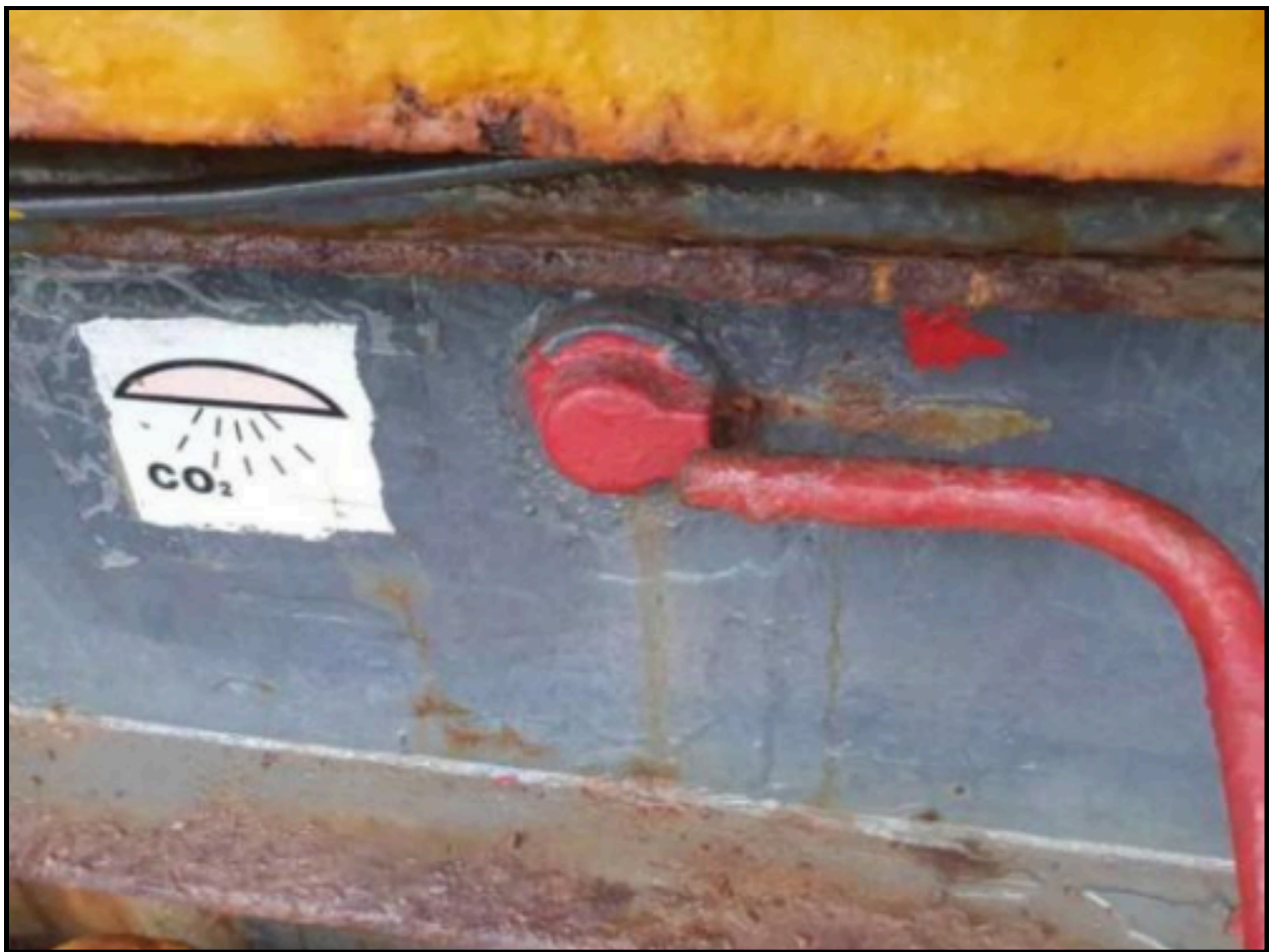
Pipe of fixed fire-extinguishing system (CO 2 ) for cargo hold cut and heavily corroded.
