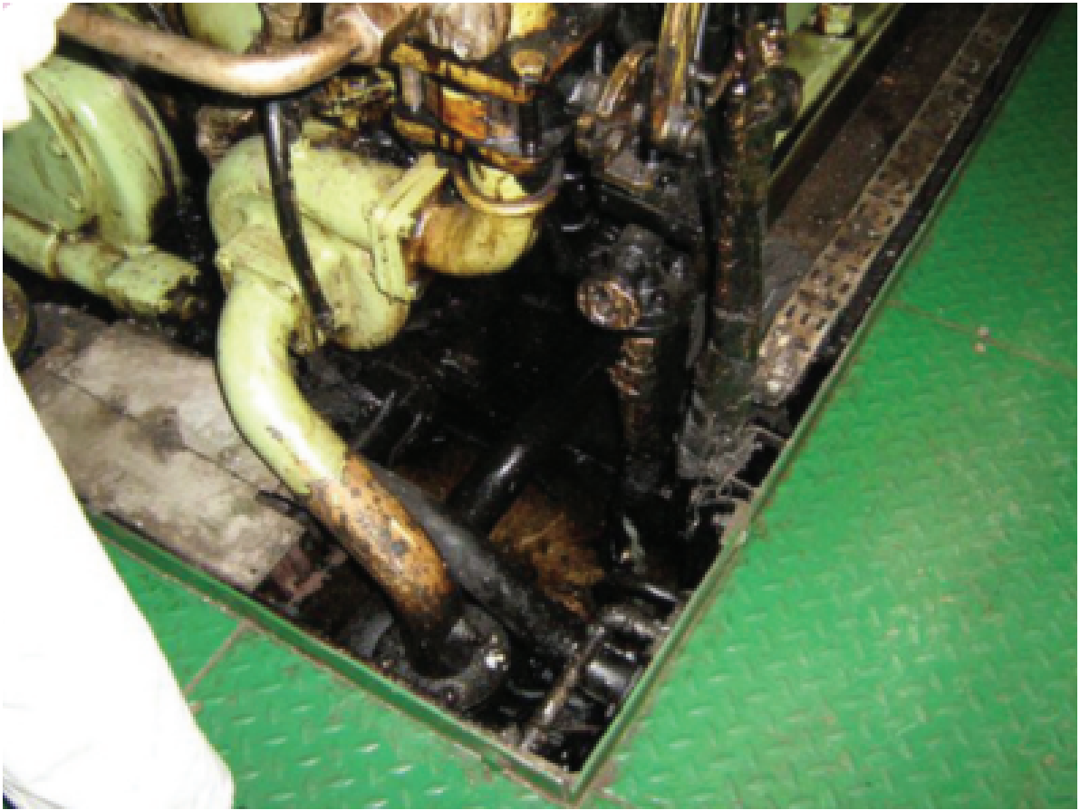
Leaking auxiliary engine
