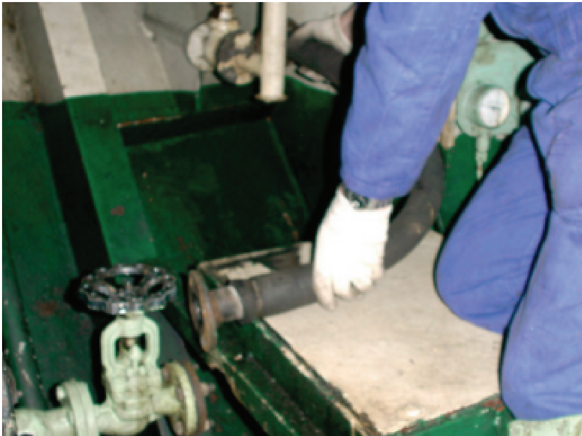
Illegal pipe - sludge pump to overboard
