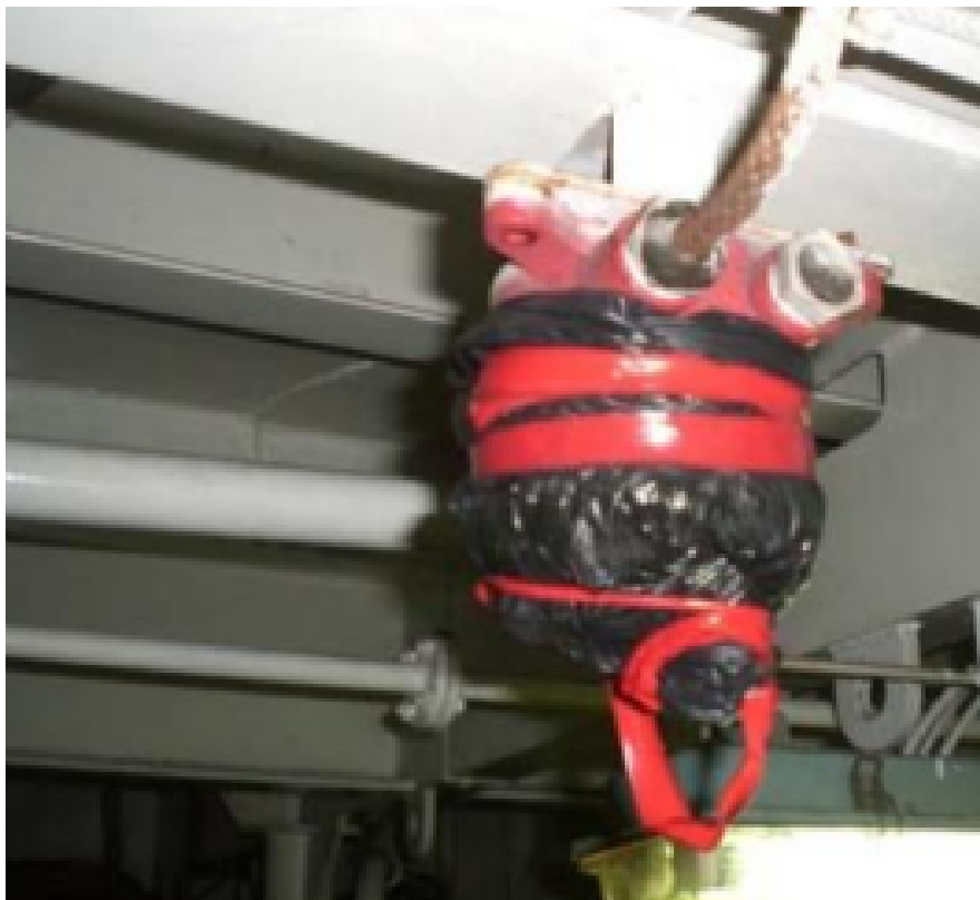
Malfunctioning smoke detector, wrapped in plastic to prevent recurring alarm sounding
