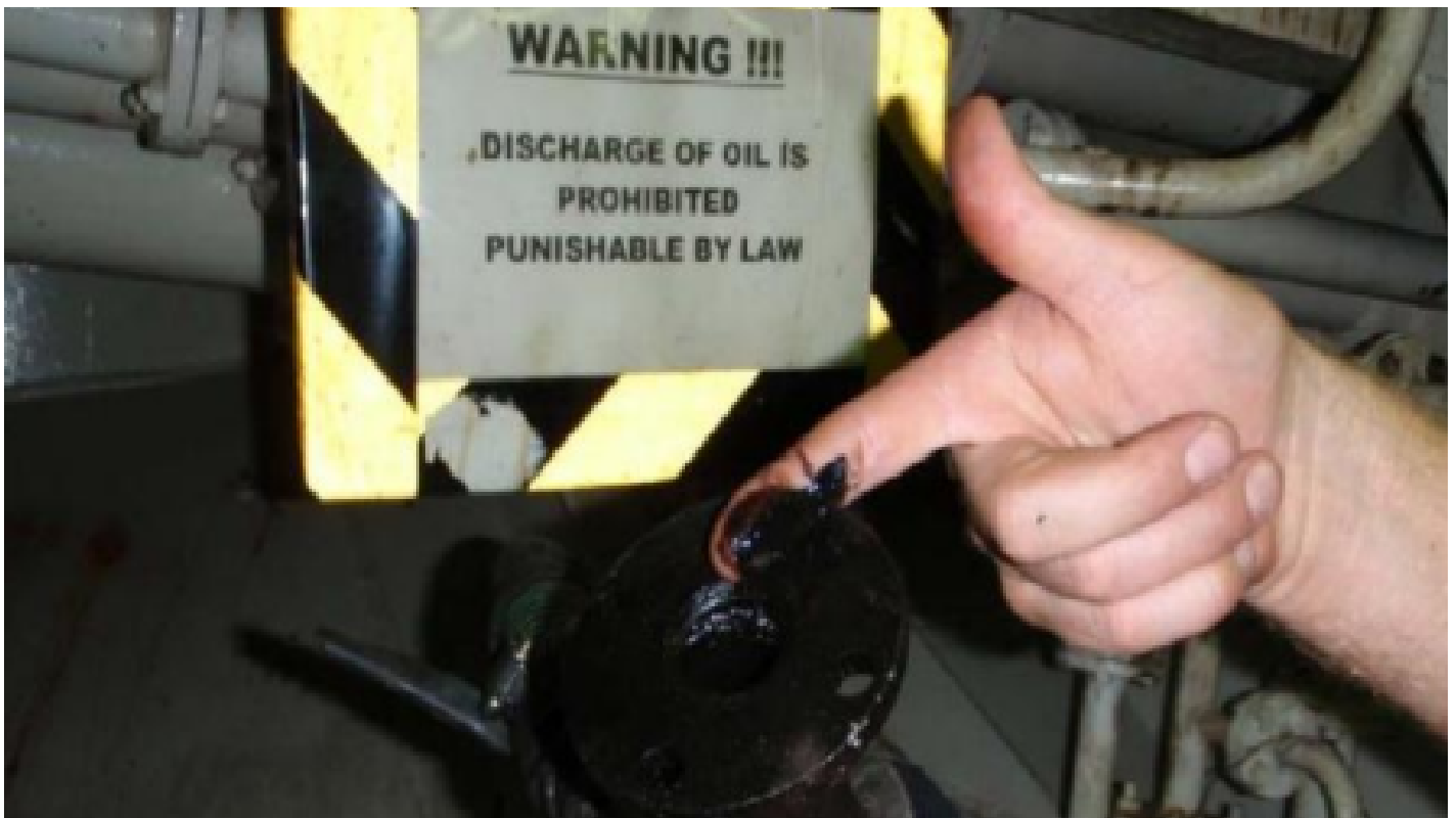
Oil on discharge side of oily-water separator
